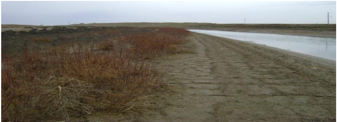
Figure 1. Deposition observed at channel station PK 205 of the Mirishkor Canal
