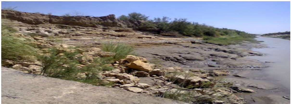
Figure 2. Erosion observed at channel station PK 310+50 of the Amu–Bukhara Machine Canal
